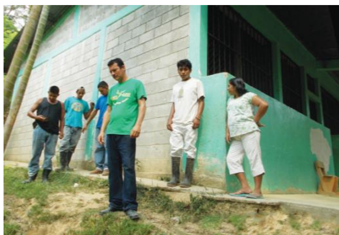
Victor and residents inspect the erosion at the school
