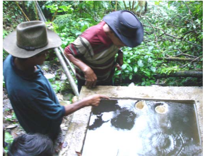
This is a sediment settlement box at a water source, from which water is piped down to a tank for distribution.
